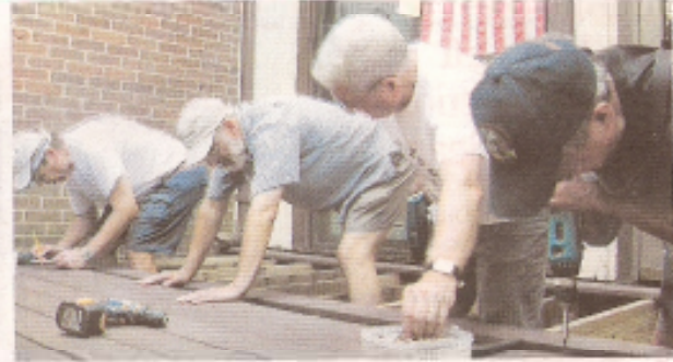
From left, Elliott Wicks, Lee Schmidt, Bob Mason and Roy Oishi, all of United Christian Parish, rebuild a deck in front of a Gabriel Home on Colts Neck Court in Reston.
